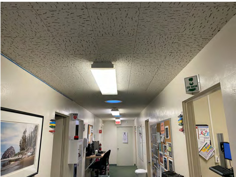
Photo 12- White Plaster Walls, White Wood Door & Casing- 2515 Main St.- CHC Area- Lead-Containing Paint & LBP (Good Condition)
