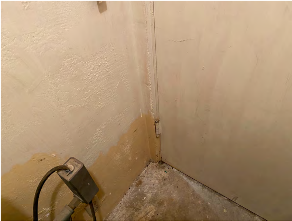
Photo 11- White/ Yellow Plaster Wall- 2515 Main St.- CHC Area- Lead-Containing Paint (Good Condition)
