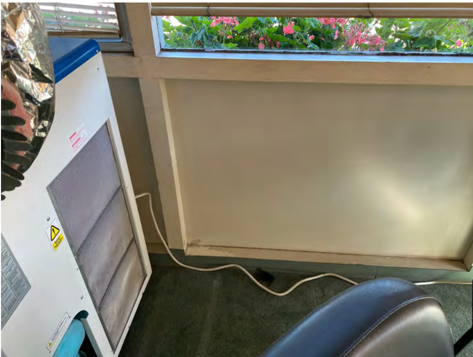
Photo 4- Transite Window Panels & White Wood Window Casing (Interior)- 2515 Main St.- CHC Waiting Room/ Exterior- ACM LBP (Good Condition)
