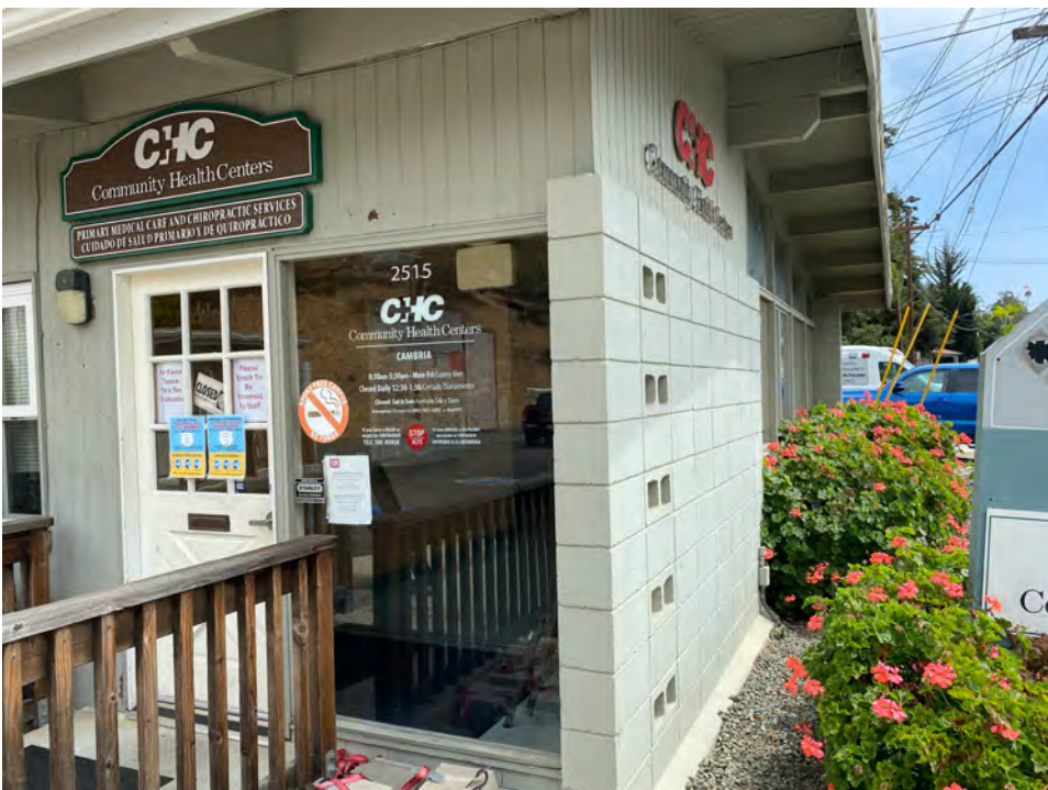
Photo 8- Gray Wood Window Casing/ Sill & Gray Wood Siding- 2515 Main St.- Exterior- LBP & Lead-Containing Paint(Poor Condition)
