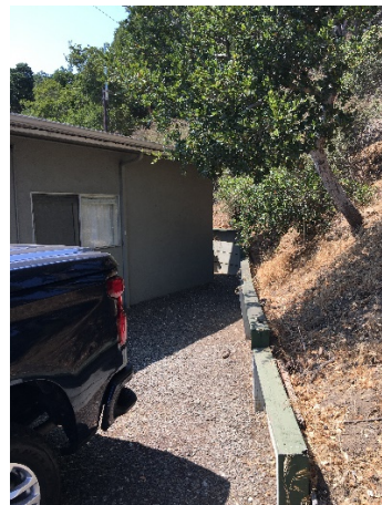
Debris wall behind facilities
