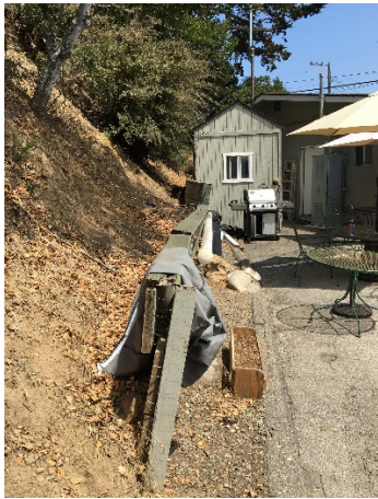
Failing debris wall
