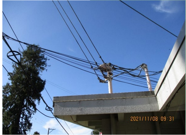
Electric service hodge-podge of wiring
