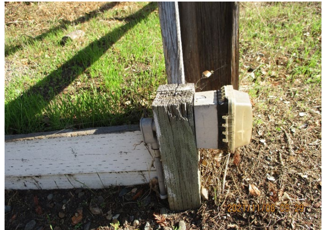
Non-compliant exterior outlet
