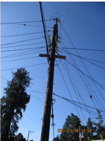
PG&E service pole
