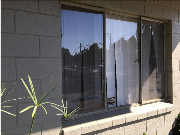
Window doesn't close properly
