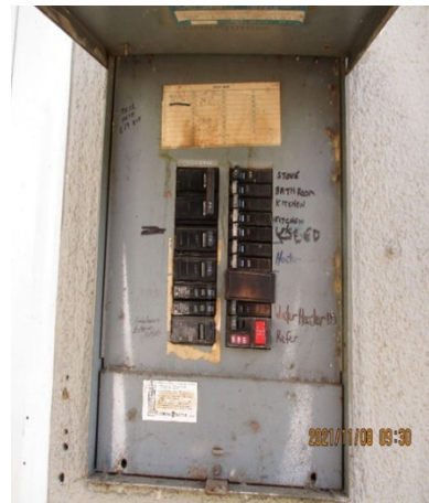
Electrical distribution panel
