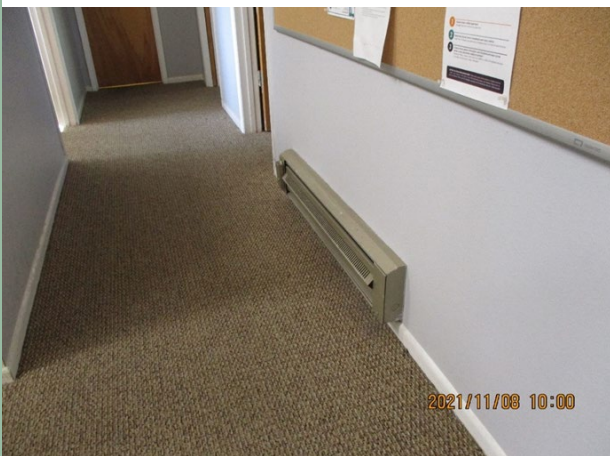
Non-working wall heater
