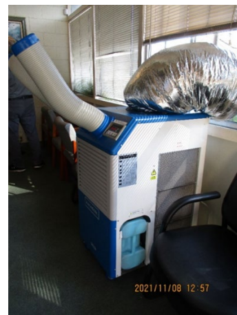
Evaporative cooler at CHC
