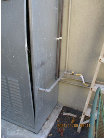
Non-compliant gas connection
