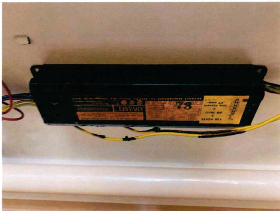
Photo 15- PCB Ballasts in Light Fixtures- 2515 Main St.- Throughout Area
