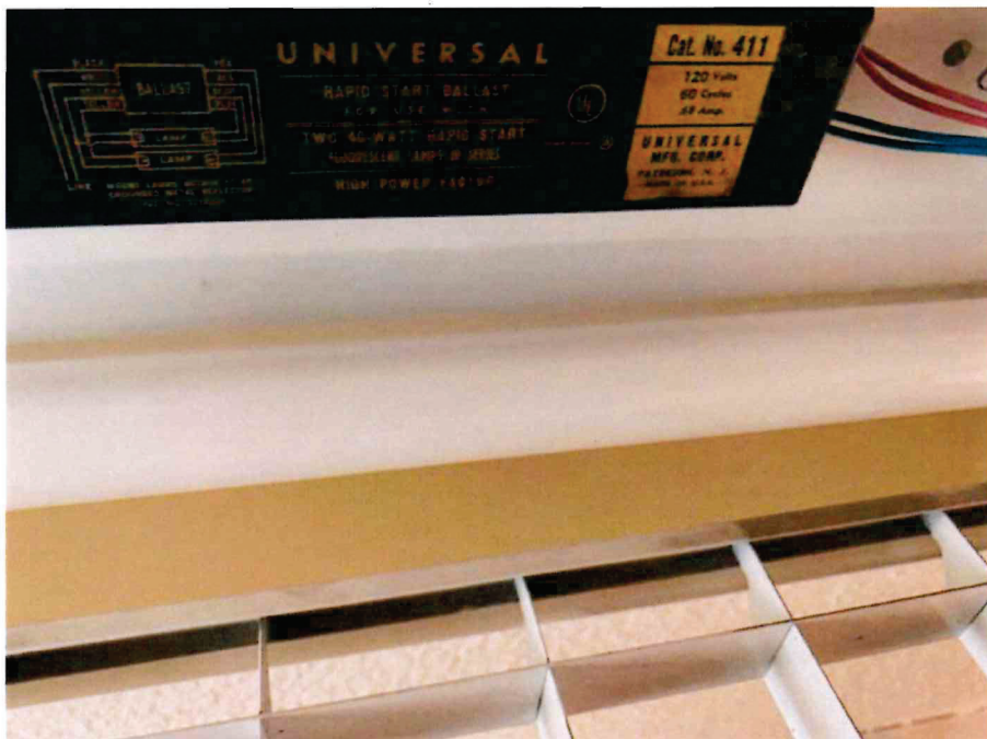
Photo 16- Mercury-Containing Light Tubes in Light Fixtures- 2515 & 2535 Main St.- Throughout Area
