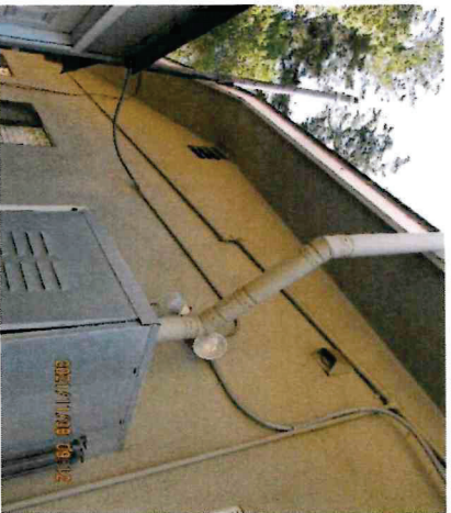
Photo 17. Gas Line Runs on side of building to DWH
