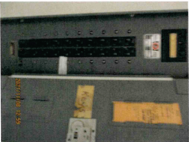
Photo 11. Power Distribution Panelboard #2
