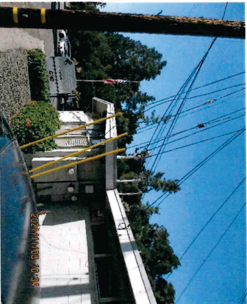
Photo 5. PG&E Laterals for four (4) Services
