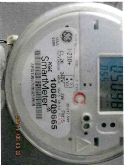
Photo 8. Multiple PG&E Meters (1 of 4 meters)
