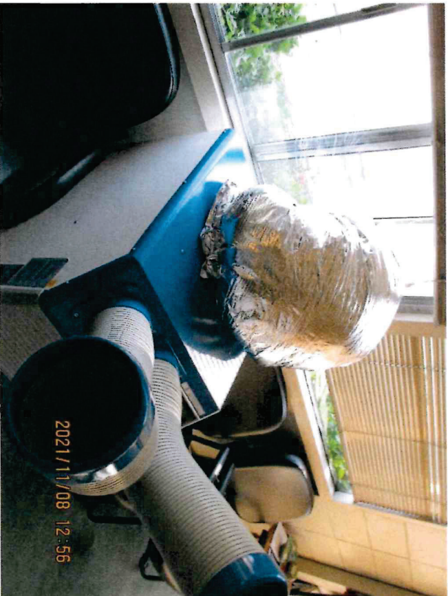
Photo 25. A Portable Evaporative Cooler – One for the Whole Building
