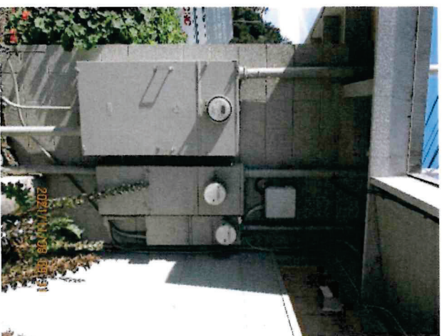
Photo 7. PG&E Services #1, 2, and 3
