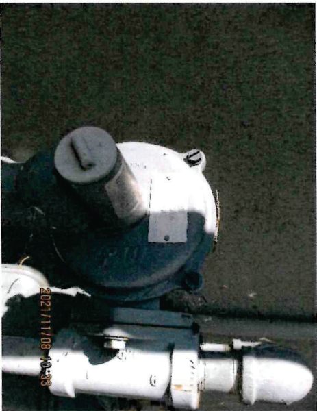
Photo 15. Gas Service Regulator
