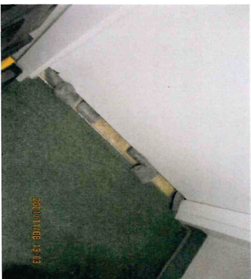
Photo 24. Steel Wool Placed Under Door
